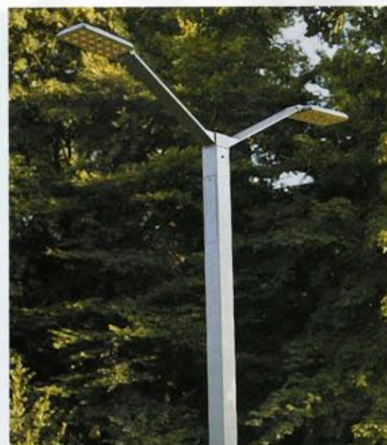
70% of Victorian street lights still use 1960s mercury vapour technology. Philips hopes its Equinox street light is the next generation lighting option.
